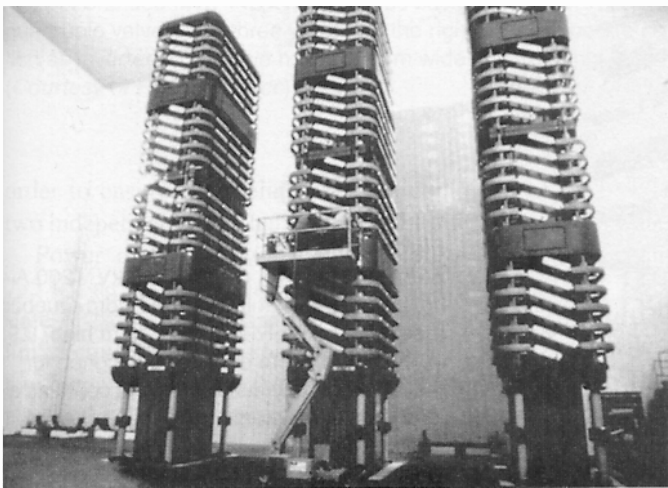
Figure 28.21b View of three quadruple valves being installed in one of the Coal Creek Terminal valve halls. Together they constitute one pole of the 400 kV system. (Courtesy of United Power Association)
